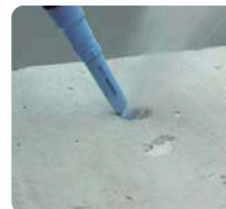
For removing drilling cuttings.
